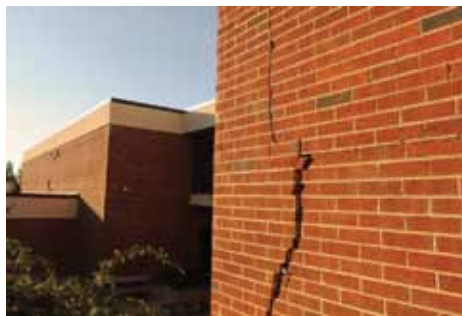
A large crack is seen in the Louisa County High School building, after being damaged by an earthquake in Mineral, Virginia.
